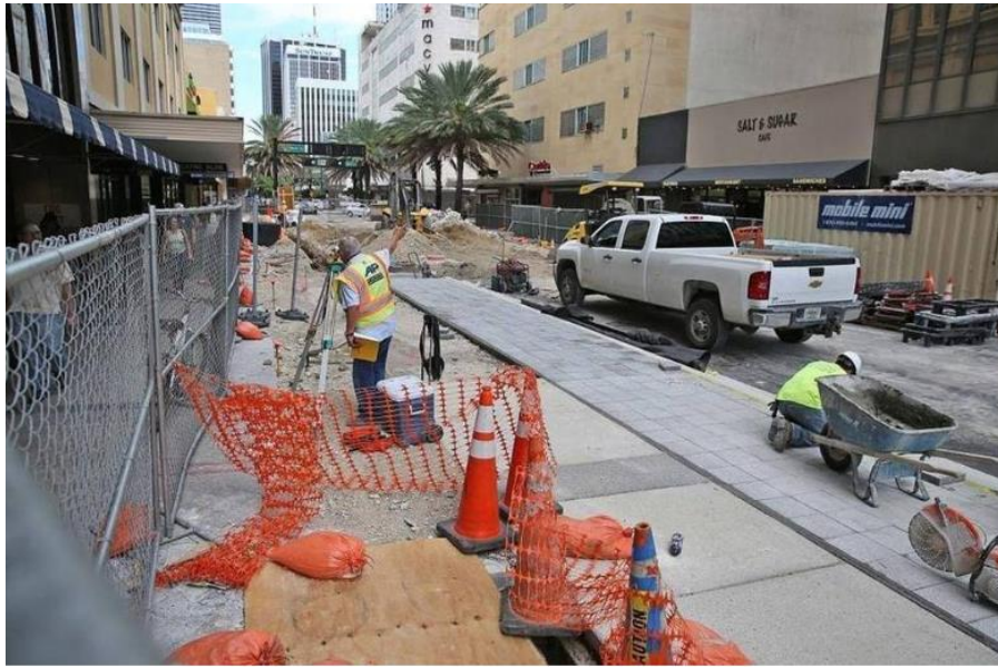
Construction crew work on the Flagler Street project which is running behind schedule as of Thursday, February 23, 2017. C.M. GUERRERO. cmguerrero@elnuevoherald.com
