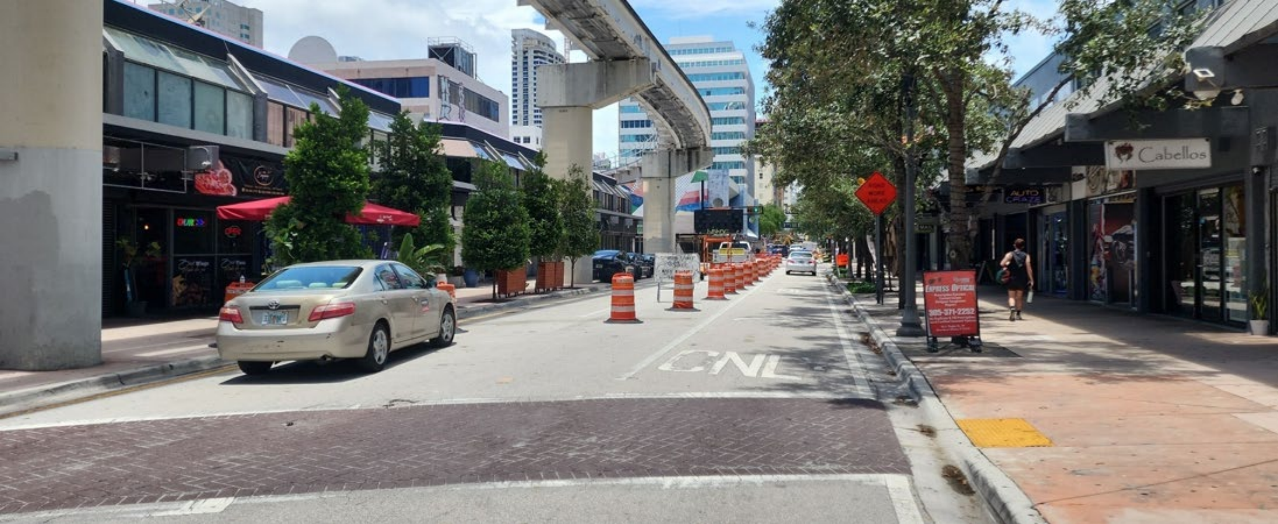
Phase D (E 1 st Ave to N Miami Ave): Maintaining MOT closure on SE 1 st Avenue.
