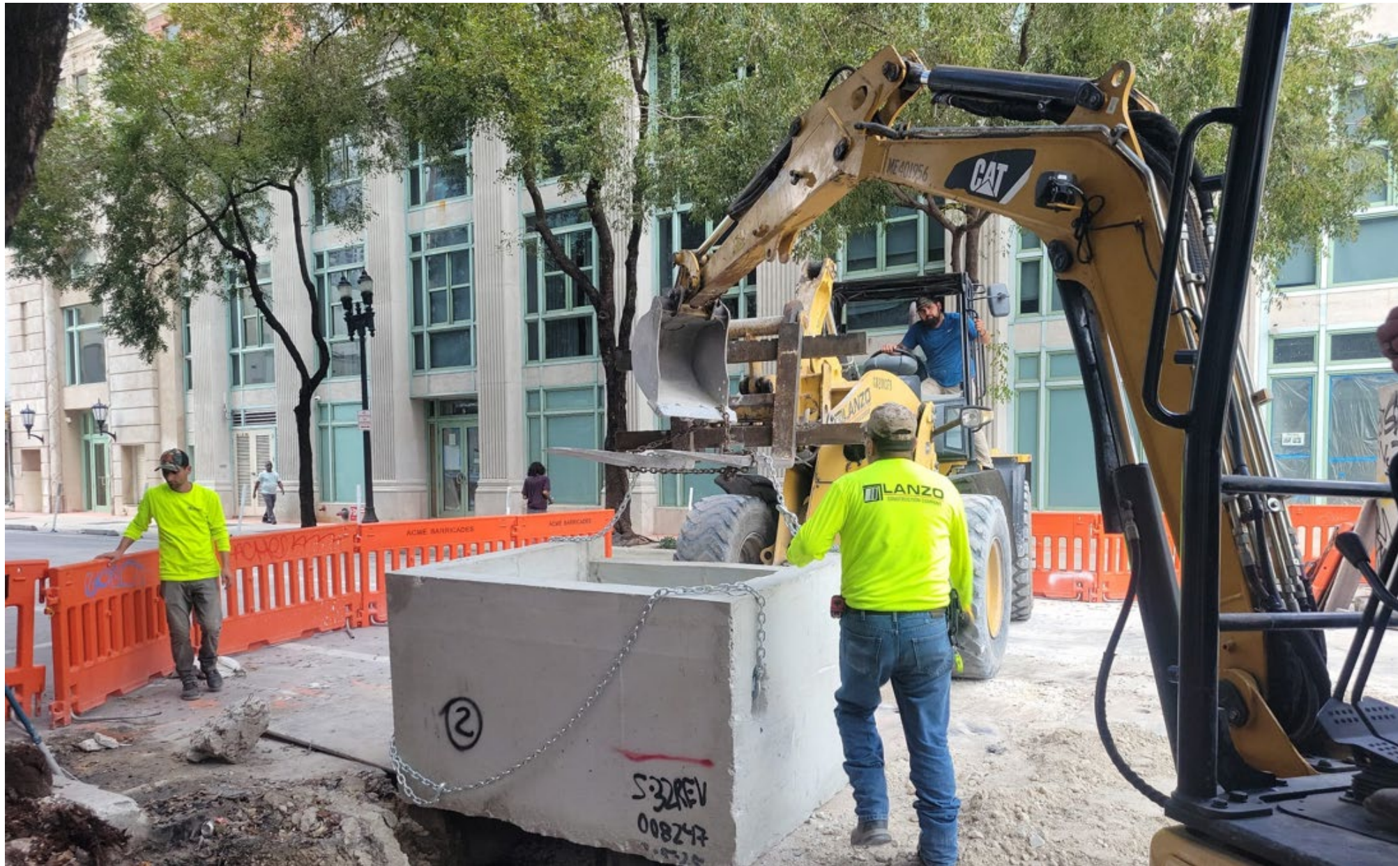
Phase D (E 1 st Ave to N Miami Ave): Installation of Drainage Structure
