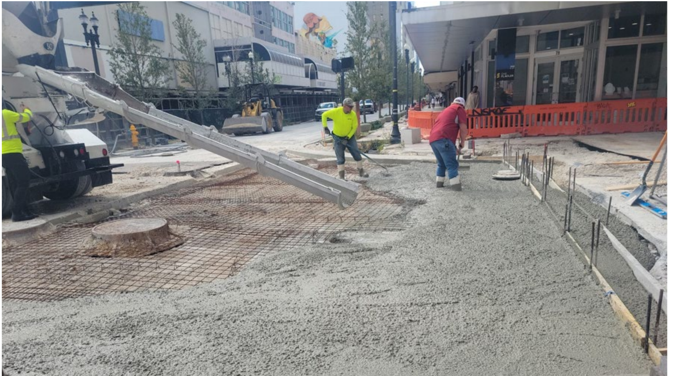
Phase D (E 1 st Ave to N Miami Ave): Concrete Pour Reinforcement for Roadway Slab
