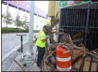
DET/NEAT Gateway Maintenance
