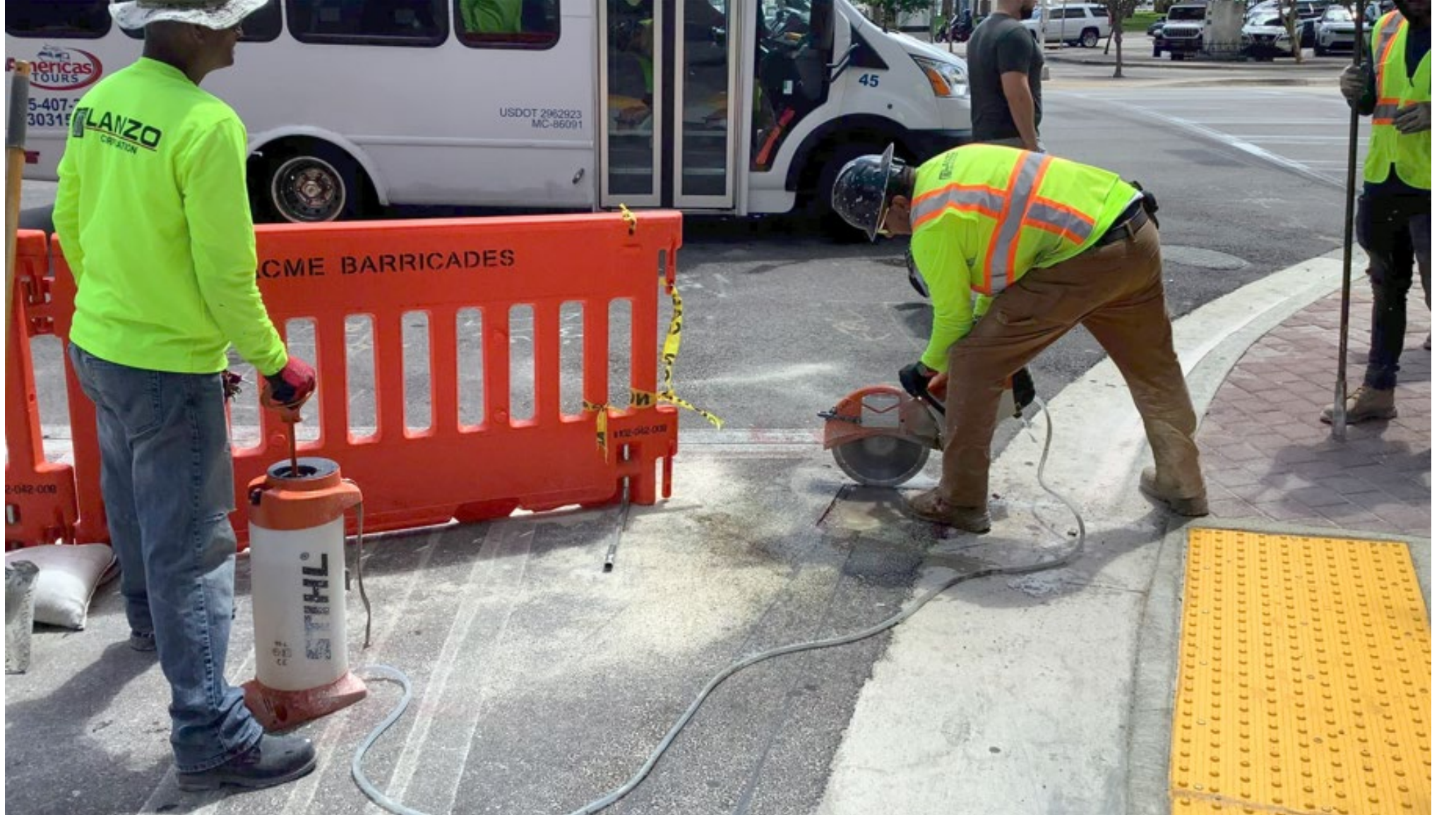
Phase A (Biscayne Blvd to E 3 rd Ave) Asphalt repair on crosswalk at Biscayne Blvd
